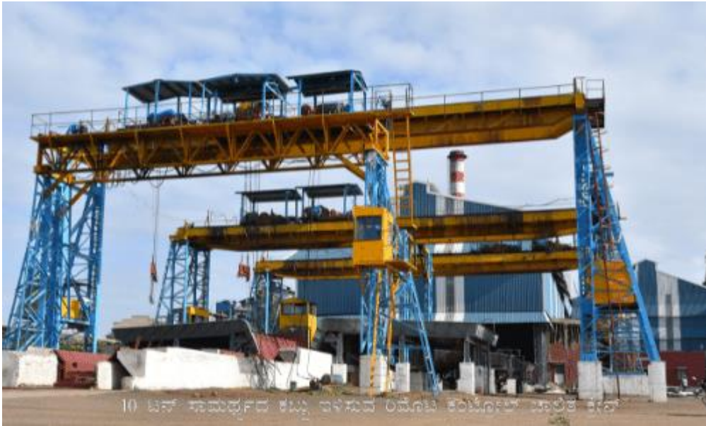
Figure 1: 10T cane unloading crane
