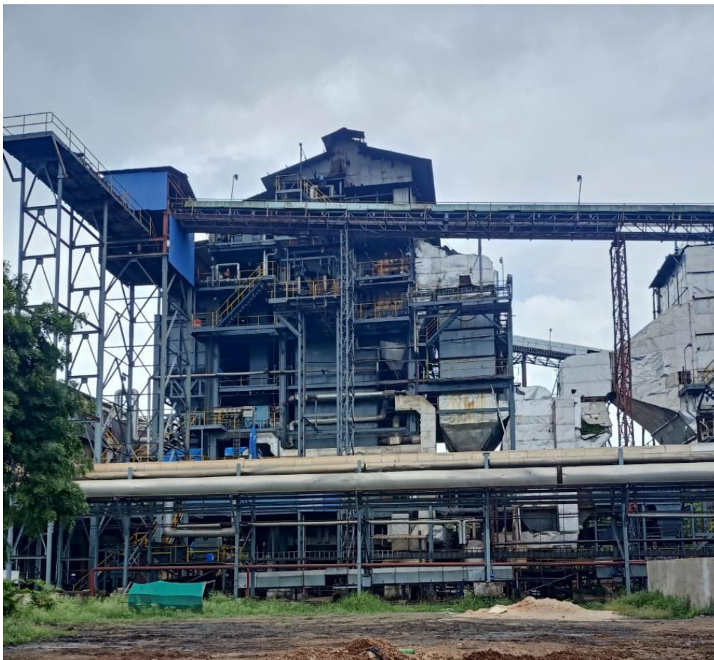
Figure 2: Overview of 150tph bagasse boiler
